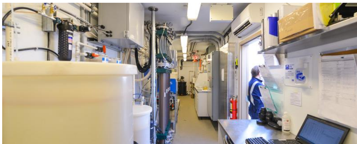
Figure 33: Selen-IX Mobile Pilot Plant (Source: Company Documents)
