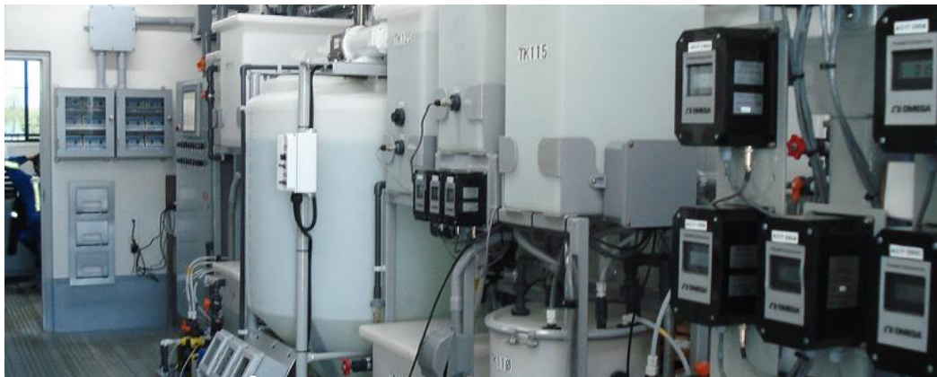
Figure 31: Sulf-IX & Sulf-IXC Mobile Pilot Plant (Source: Company Documents)
