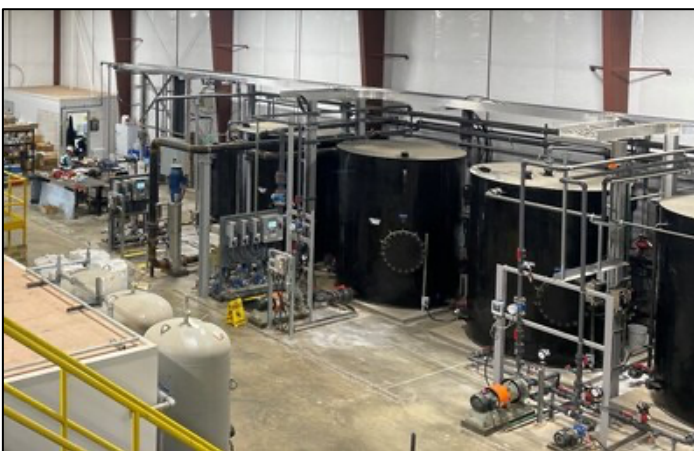
Figure 3: Selen-IX Plant at Wharf Mine (Source: Company Documents)
