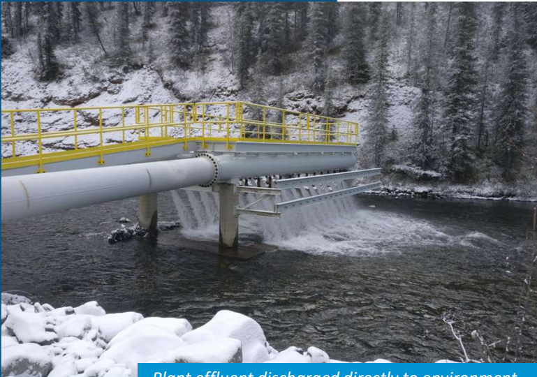
Plant effluent discharged directly to environment
